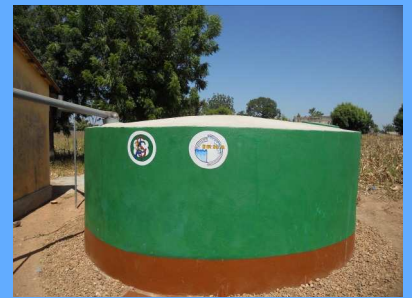
New rainwater tank in Togo
